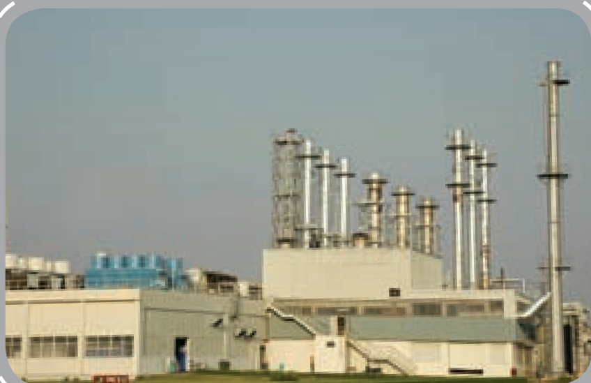
Captive power plant using clean fuel natural gas
