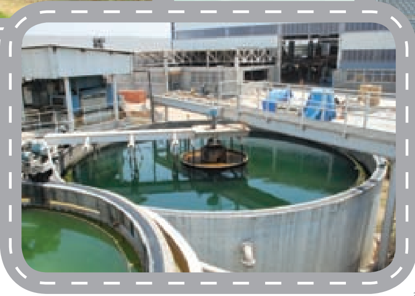
An effluent treatment plant
