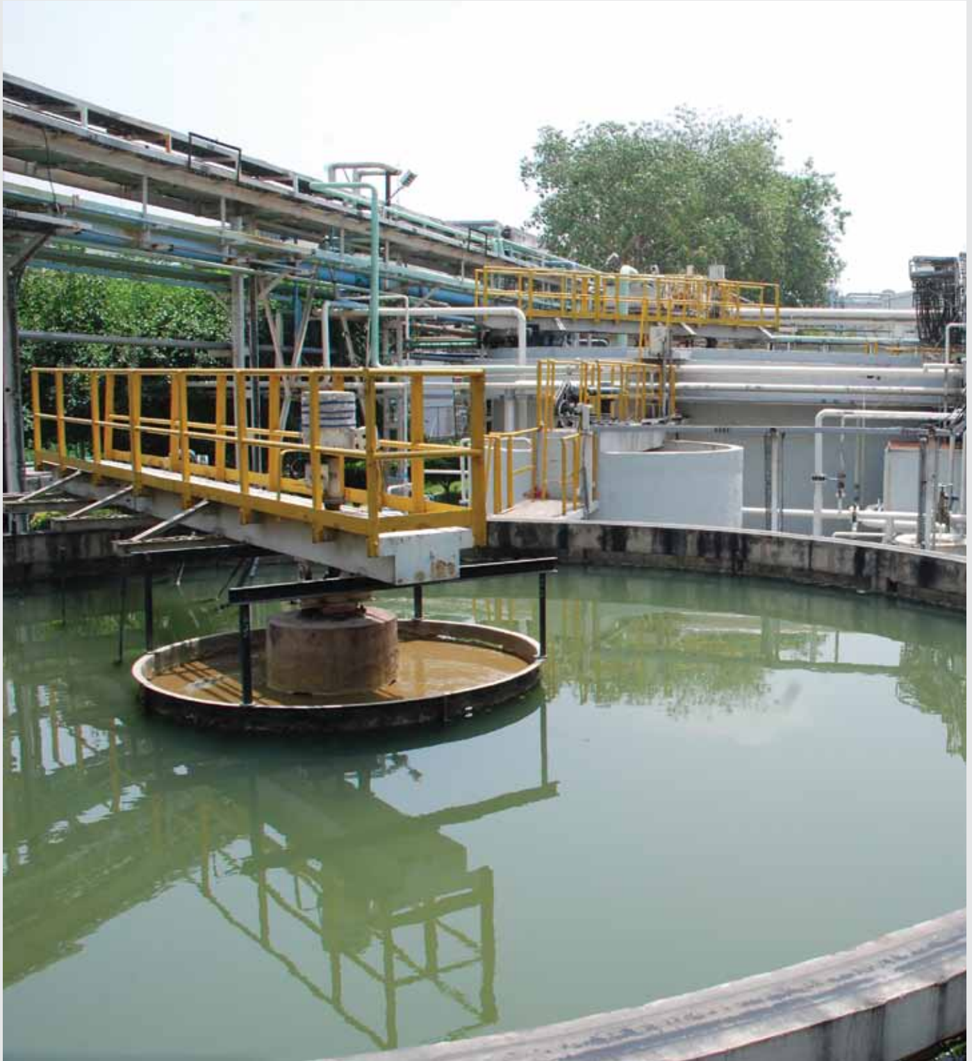
Effluent Treatment Plant at the Gurgaon facility.
